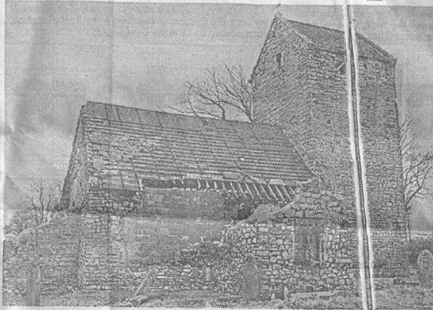
St Mary's Church — shortly after it was wrecked by vandals in April.
